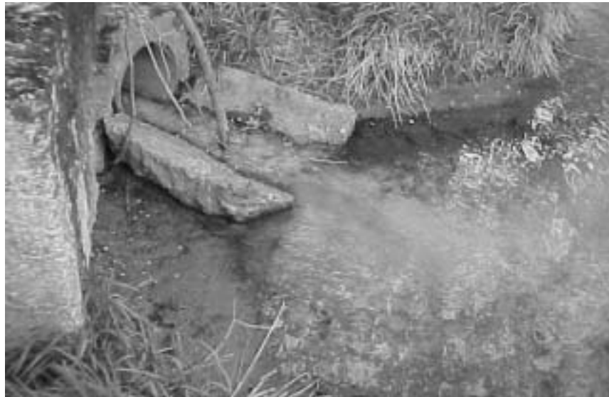
RCAP's projects focus on eliminating raw sewage discharges like this one in Rush County. In many areas, wastewater flows untreated from homes and businesses. Untreated wastewater can cause nutrient pollution, spread pathogens, cause fishkills, and lead to a whole host of other problems.
